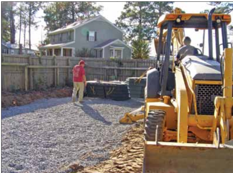
LEFT: Bron Bradley from Anua helps guide the second 150 gpd Puraflor peat biofilter into position. BELOW: Brian Lucas of Lucas Soil Evaluation finishes the gravel bed for the direct-discharge peat biofilters.
