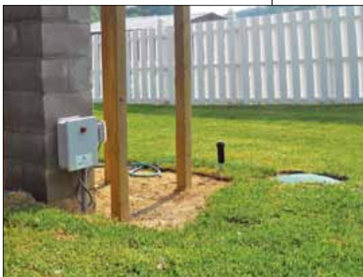
The Aquaworx IPC control panel is installed on a pillar. The septic tank riser is to the right.
